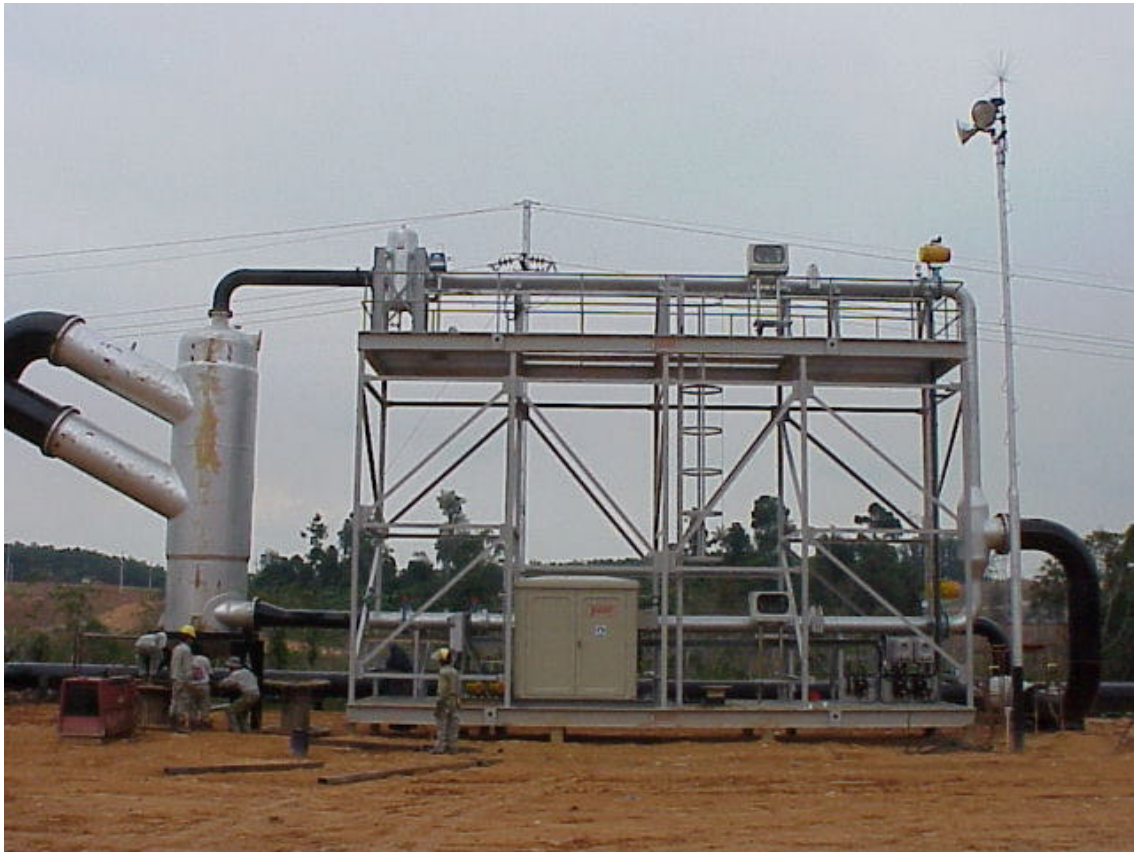
Figure 2: World's Largest GLCC Commissioned by Caltex Pacific Indonesia (CPI)
